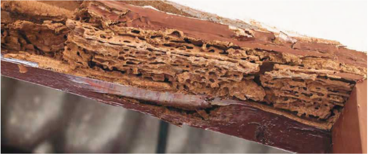
Termite damage to wood
